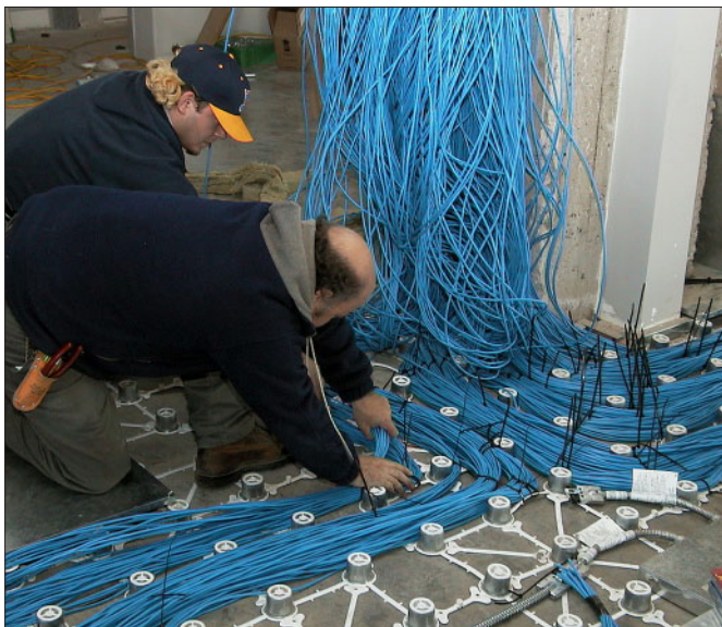
Calgary, Alberta-based Critical Mass uses miles of data cables for its Web design and Internet consulting business. Cables are run in a Haworth/SMED access floor.
